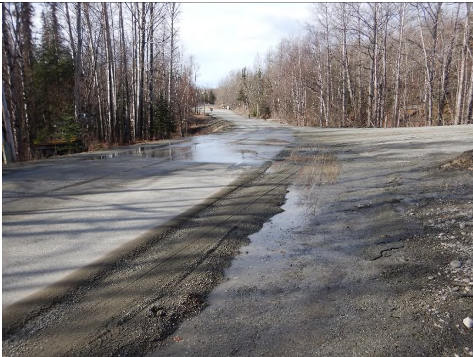
Roadway ponding at Wilderness Drive.
