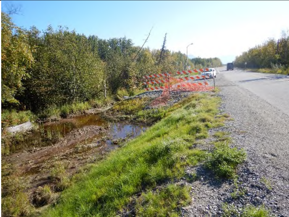
Ineffective BMPs at Nelson Drive.
