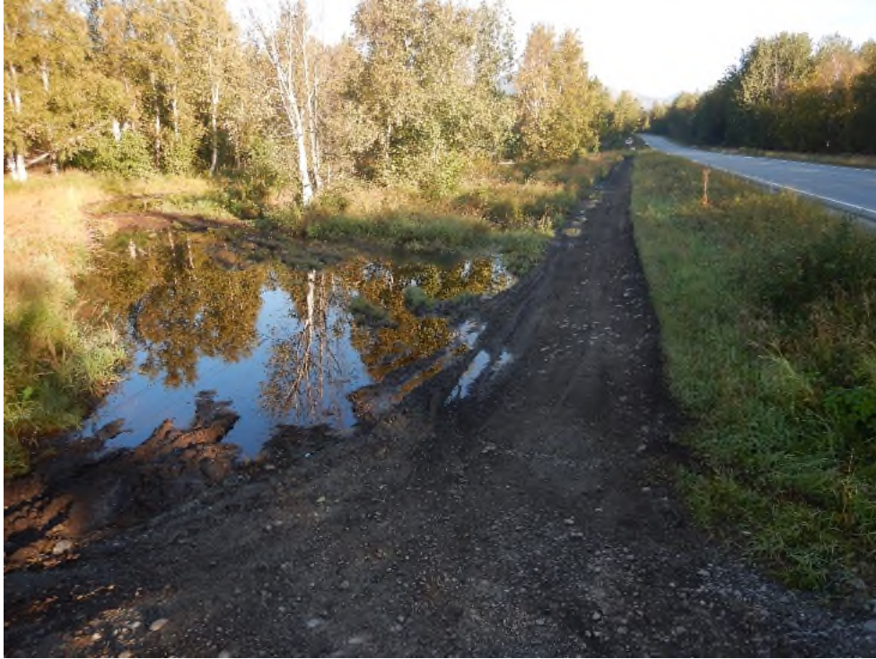
Roadside ponding at north side of driveway and in ATV trail.
