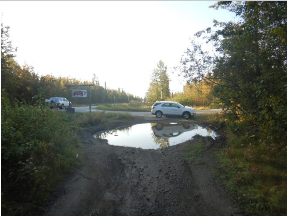
Roadside ponding at north side of road and in ATV trail.
