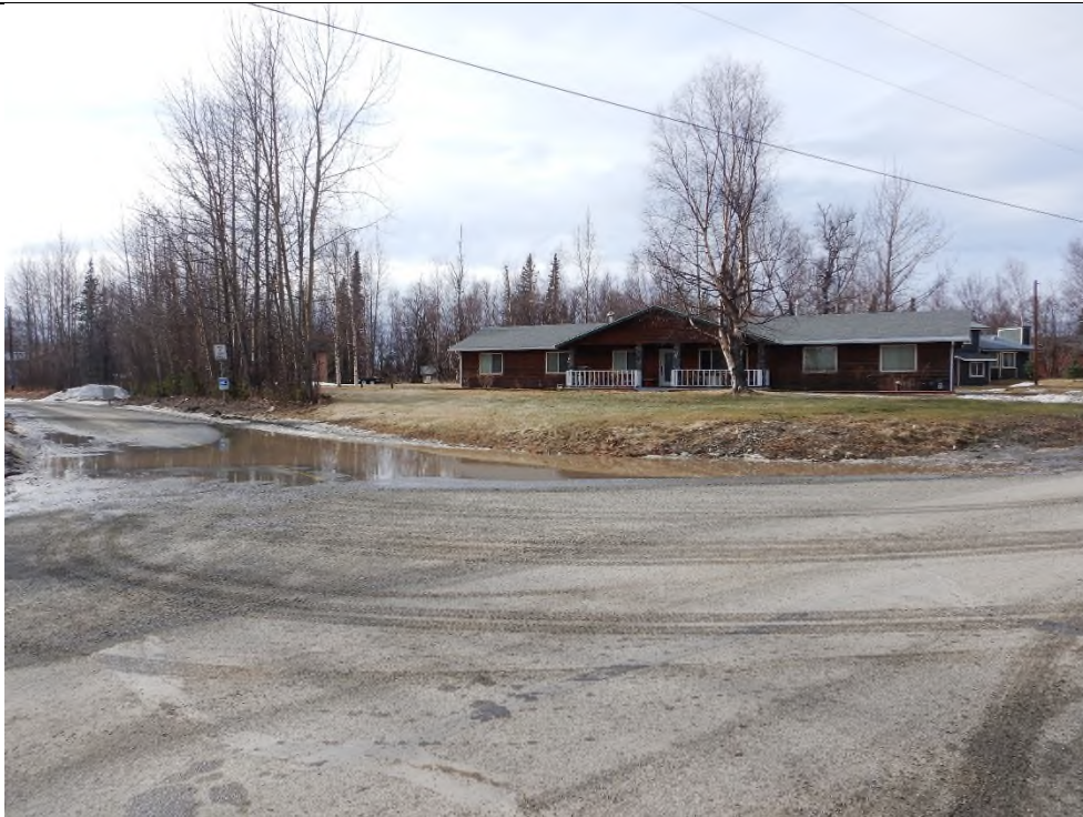
Ponded water in roadway at the corner of Tern Drive and Dove Lane.
