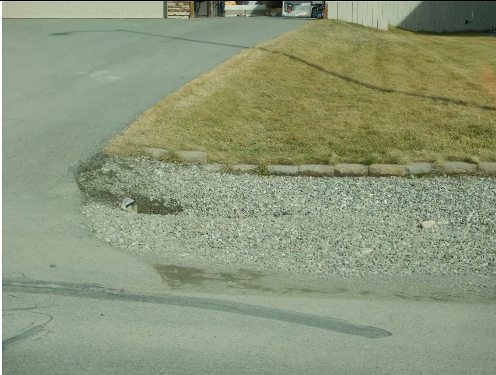
Crushed driveway culvert along Fetlock Drive.
