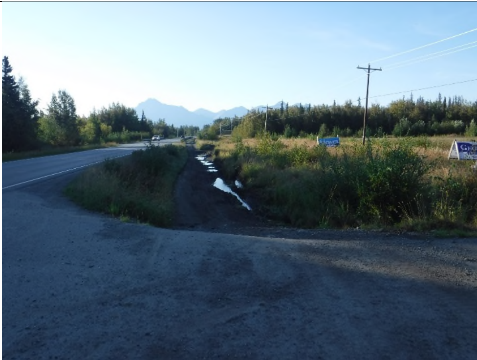
Roadside ponding at south side of driveway in ATV trail
