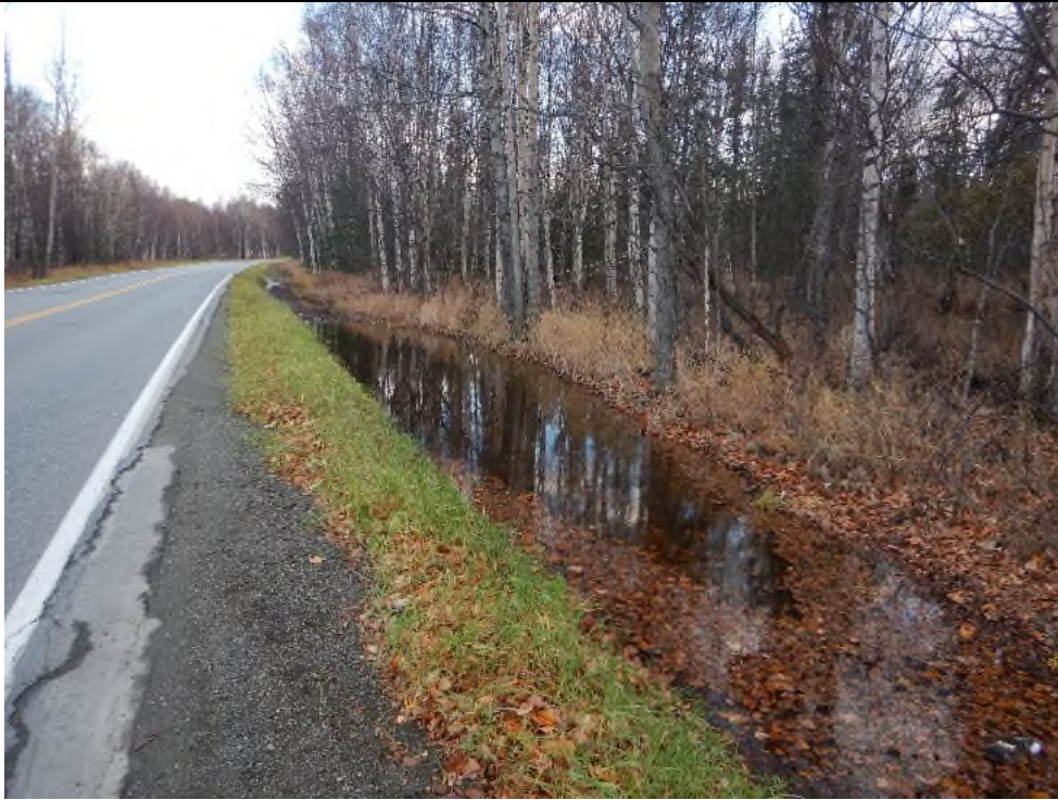
Ponding in ditches/ATV trails along Stringfield Road.
