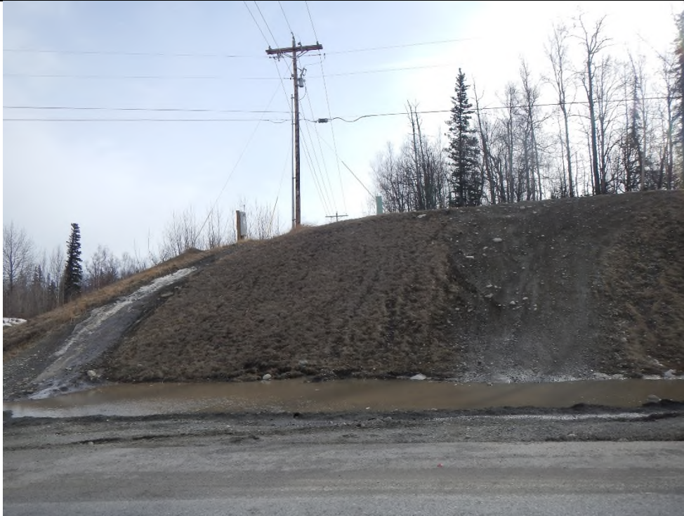
Ponding along Trunk Road.
