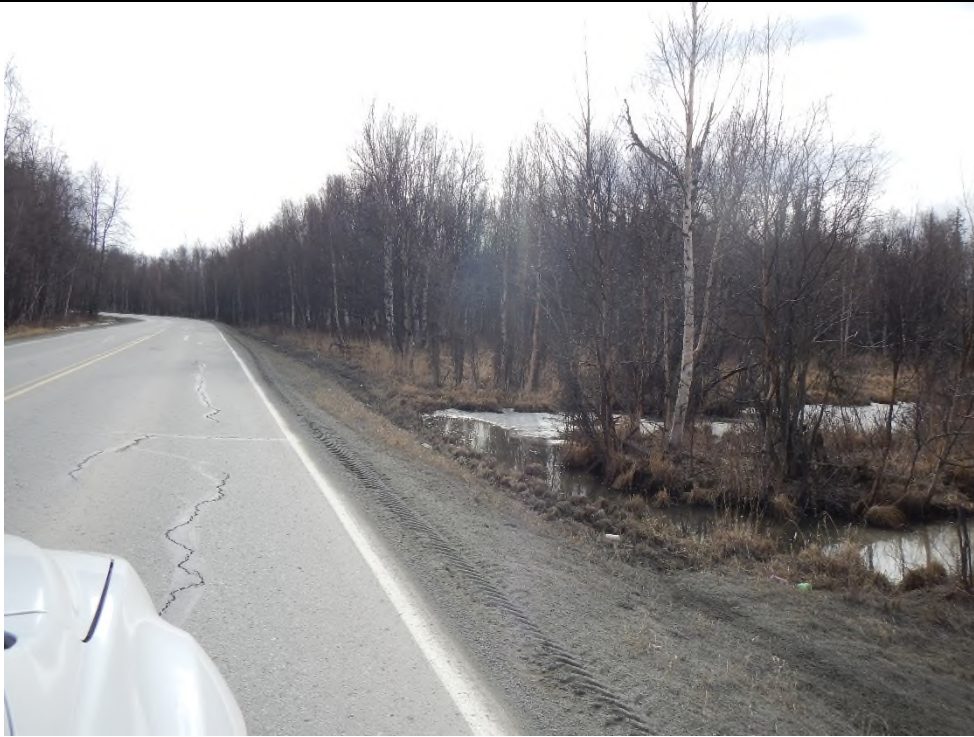
Wasilla Creek encroachment at Stringfield Road.
