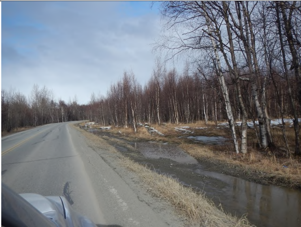
Ponding in ditches/ATV trails along Stringfield Road.
