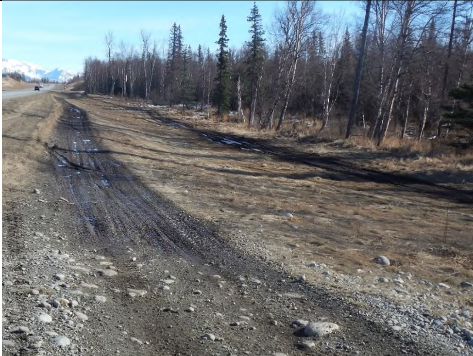
Ponding in ATV trail on east side of Trunk Road looking north.
