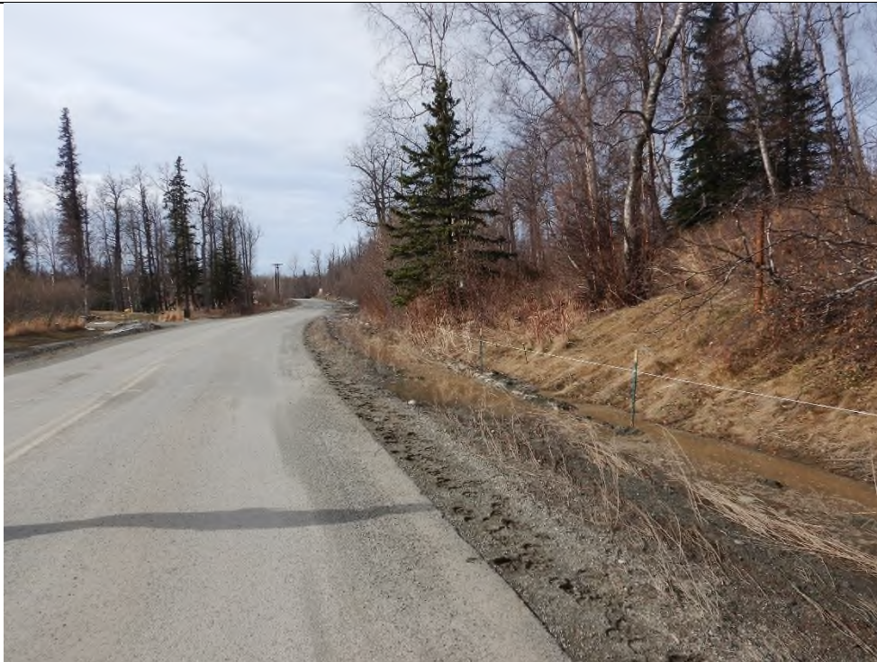
Standing water in shallow ditches along Tern Drive.
