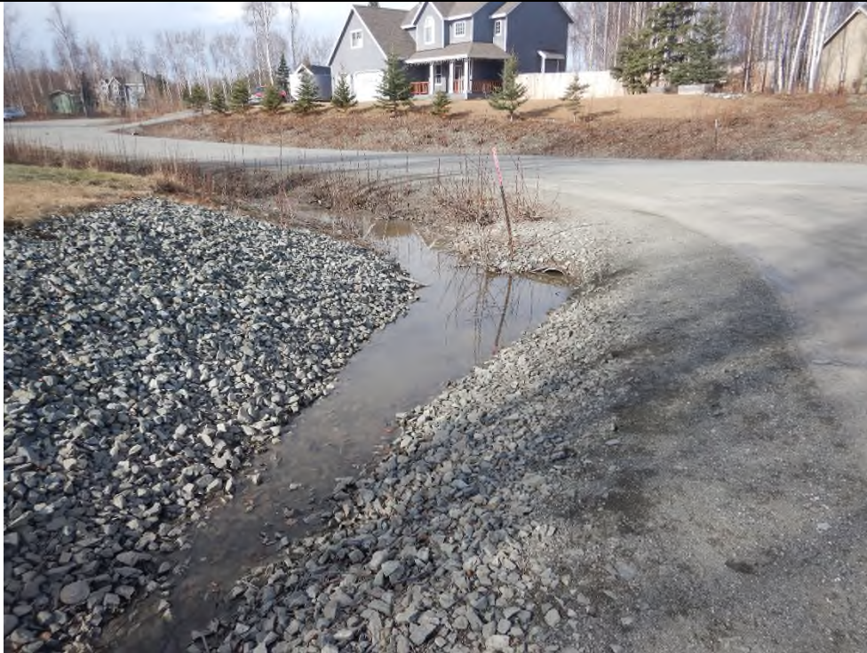
Submerged culvert at Bit Circle.
