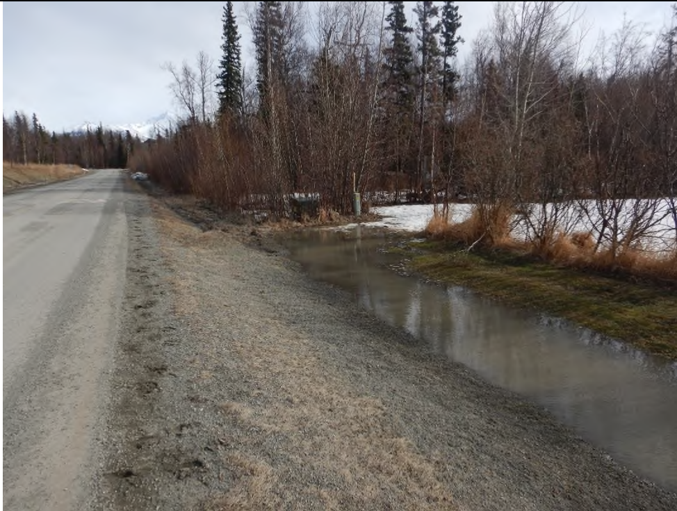
Ponding in ditches along Tern Drive near utilities.
