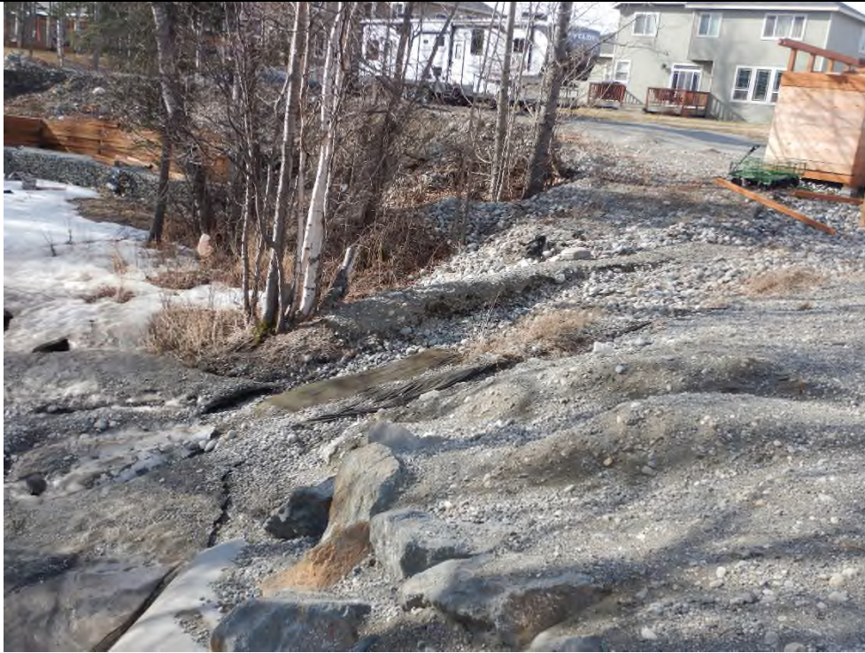
Sediment contamination and erosion at Wasilla Creek culvert on Fetlock Drive.
