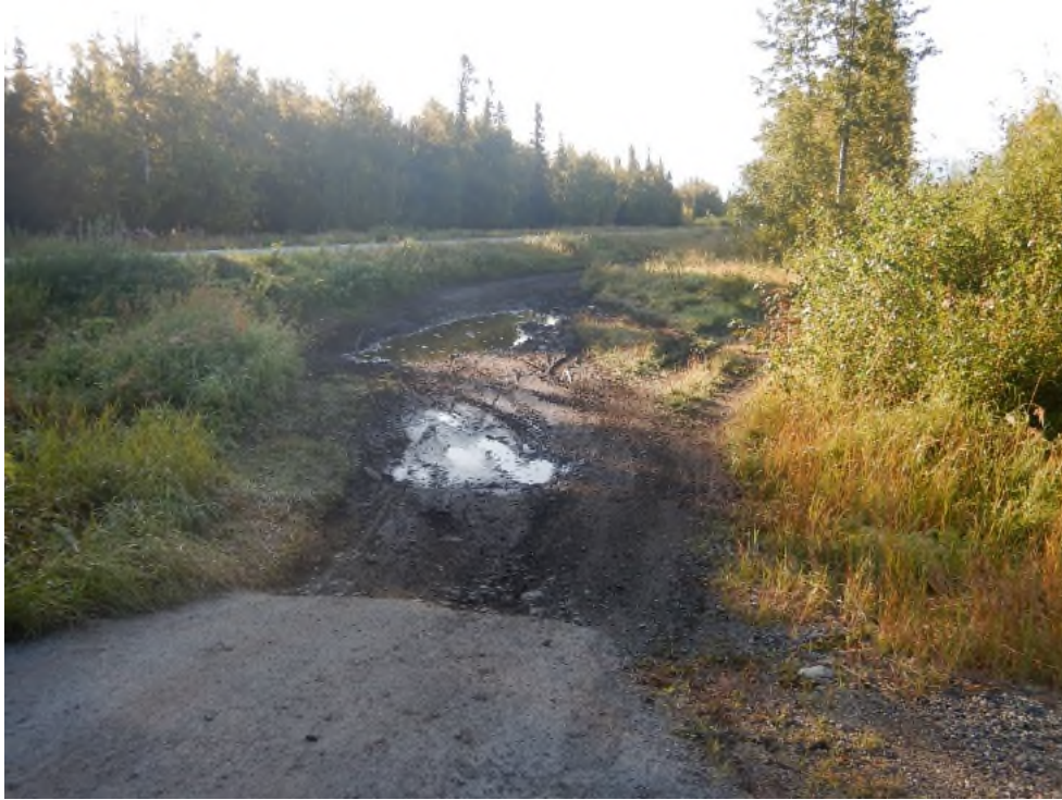
Roadside ponding at south side of road and in ATV trail.
