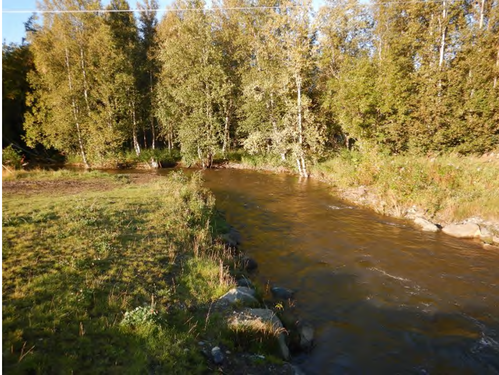
Wasilla Creek downstream streambank erosion at bend.
