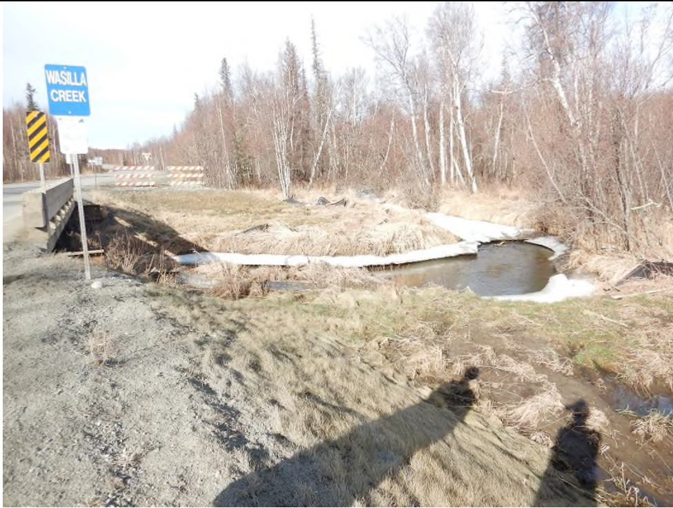
Sediment contamination at Wasilla Creek crossing at Nelson Drive.
