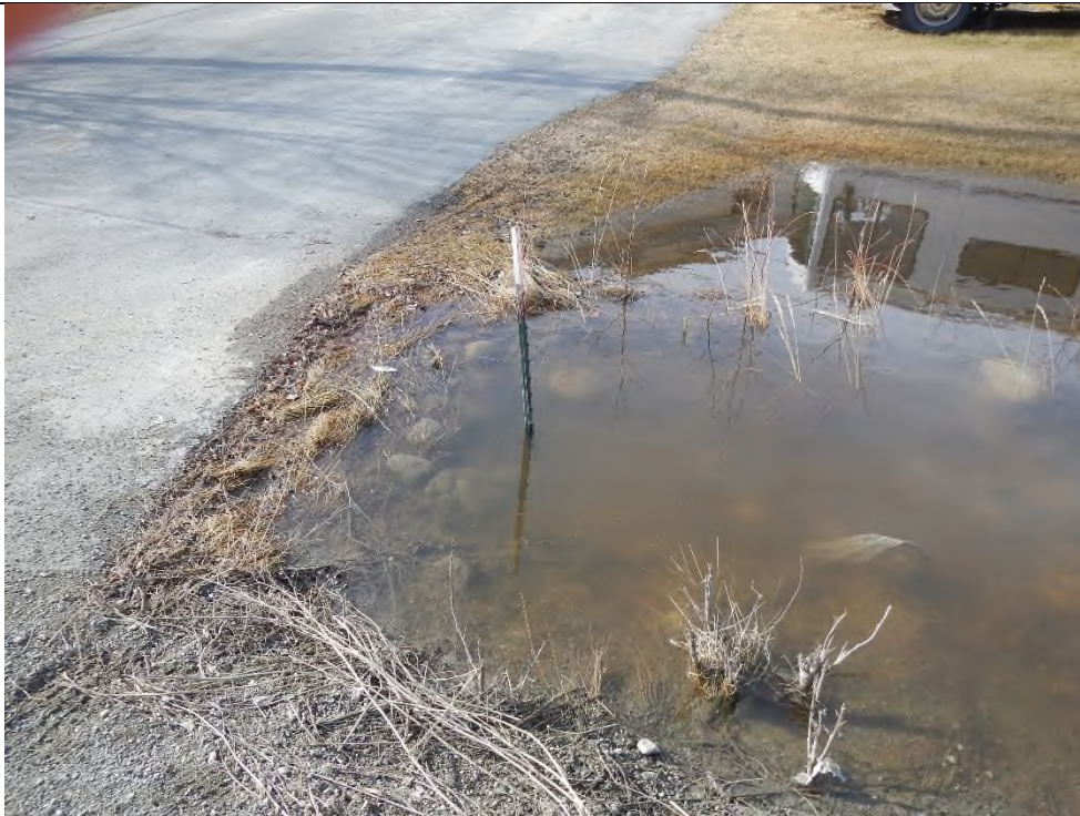
Blocked driveway culvert at Vickie Circle.
