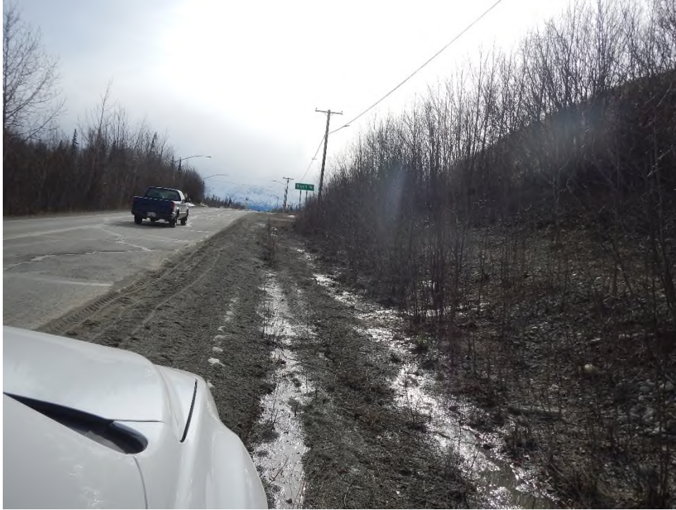
Ponding in shallow ditches/ATV trails along North 49th State Street.
