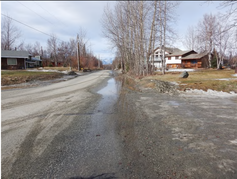
Standing water in roadway at Tern Drive.
