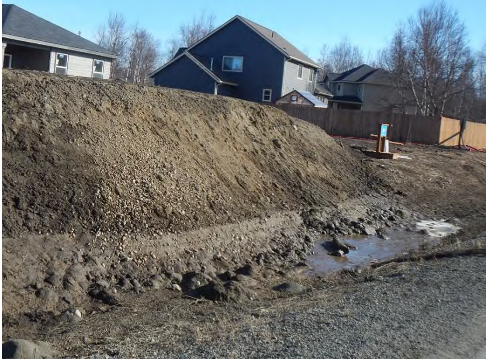
Corner of Commons and Tributary Avenue – looking east. Residential storage of large amount of material without BMPs.
