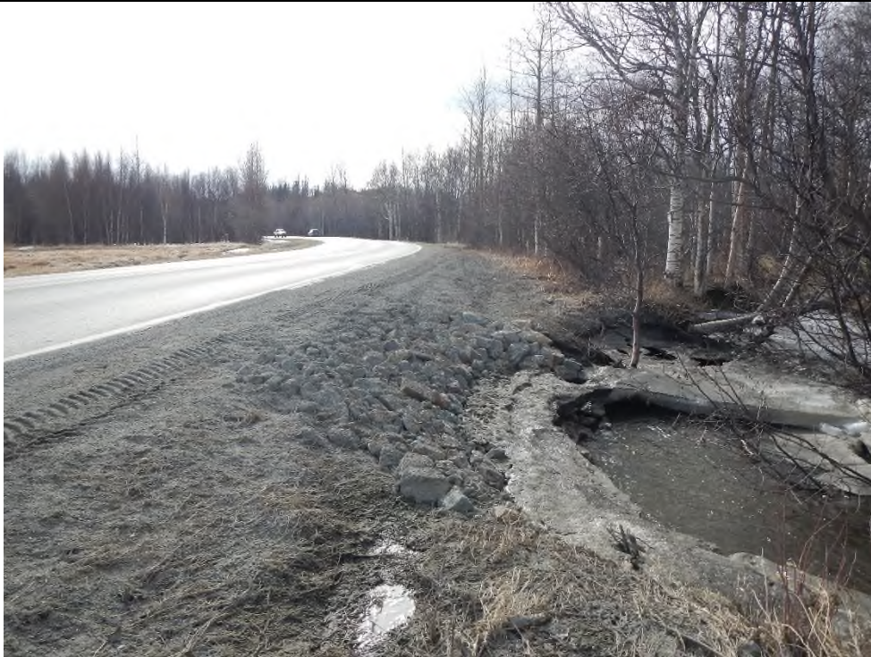
Wasilla Creek encroachment and sediment contamination at Stringfield Road.
