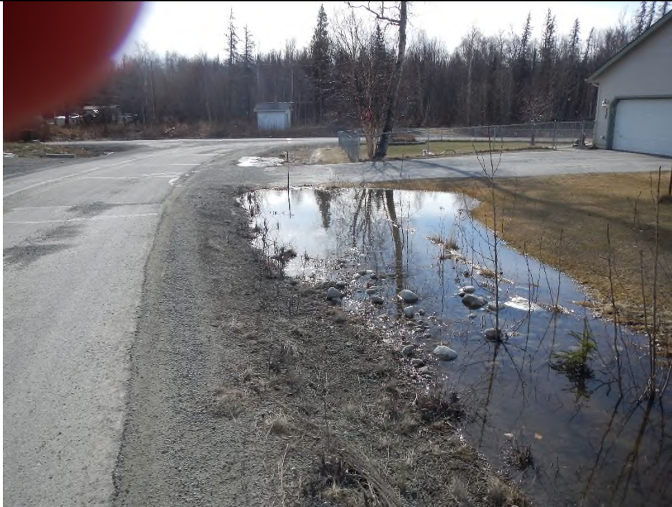
Blocked driveway culvert at Vickie Circle.
