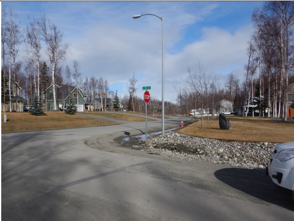
Submerged culvert at Bit Circle.
