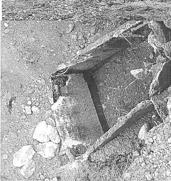
1119 E. Casney Destroyed Septic Tank
