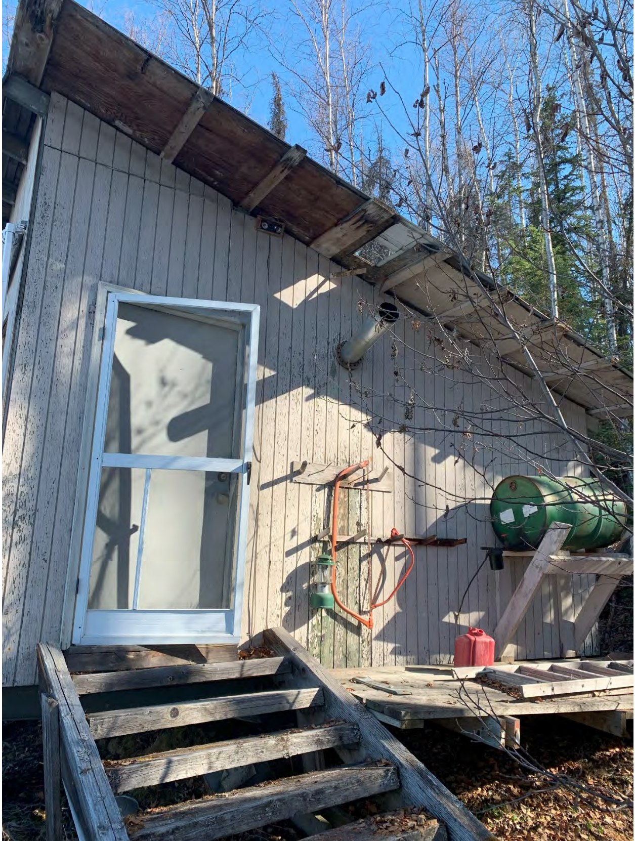
Pointing northeast. Showing the south side of the cabin, which is the entrance.
