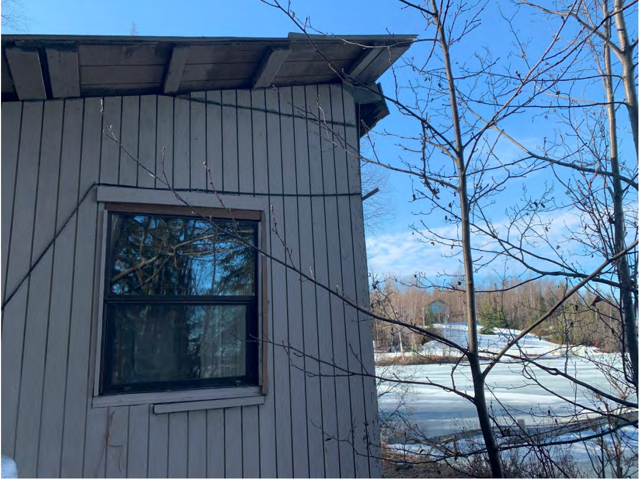
Pointing south. Showing the northwest corner of the cabin and Big Lake beyond.
