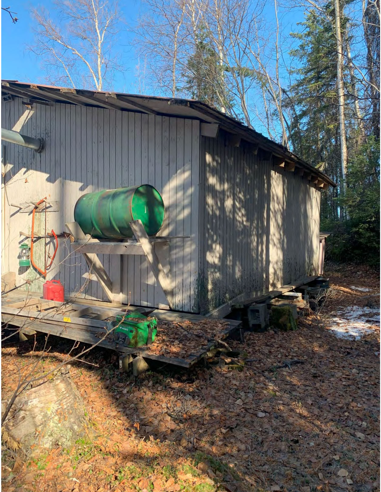
Pointing north. Showing the south and east sides of the cabin. The oil barrel is empty and has not been used for years, according to the owner.
