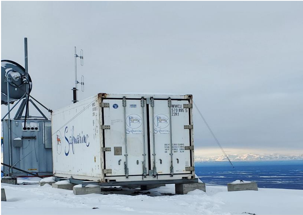
Above Photo: New Montana Mountain Telecom Site
