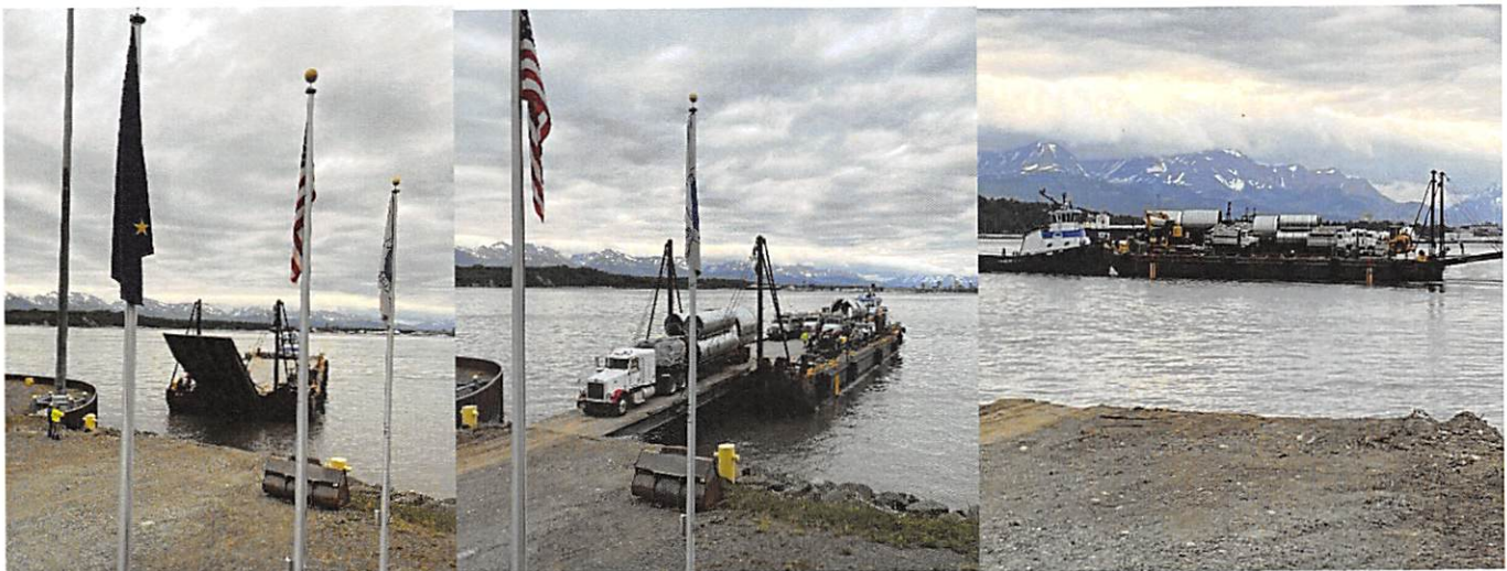
Above Photos: June 8 th 5:44 AM: Western Construction arrived with Barge PT&S379. 6:12 AM: The barge was safely loaded and headed to Tyonek with 275 tons of heavy equipment and project cargo.
