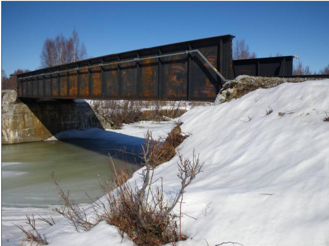
Photograph C- 6: West side of Little Susitna River Bridge (ANC-00085) looking north (Segment 6; May 2012)
