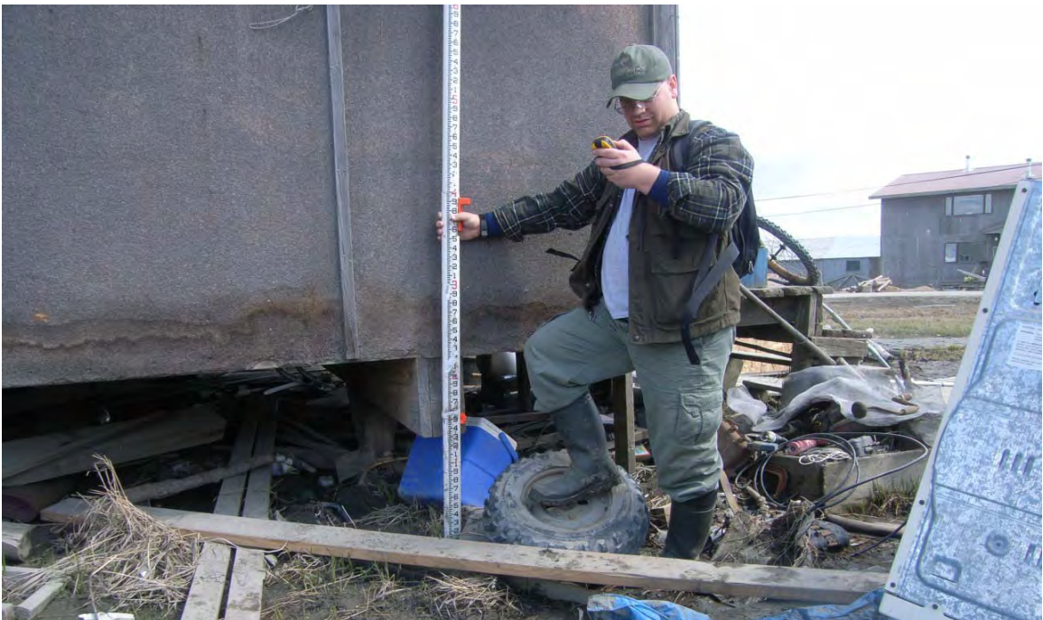
Figure 8: Water stain on wood siding, Emmonak, Poor, 2009
