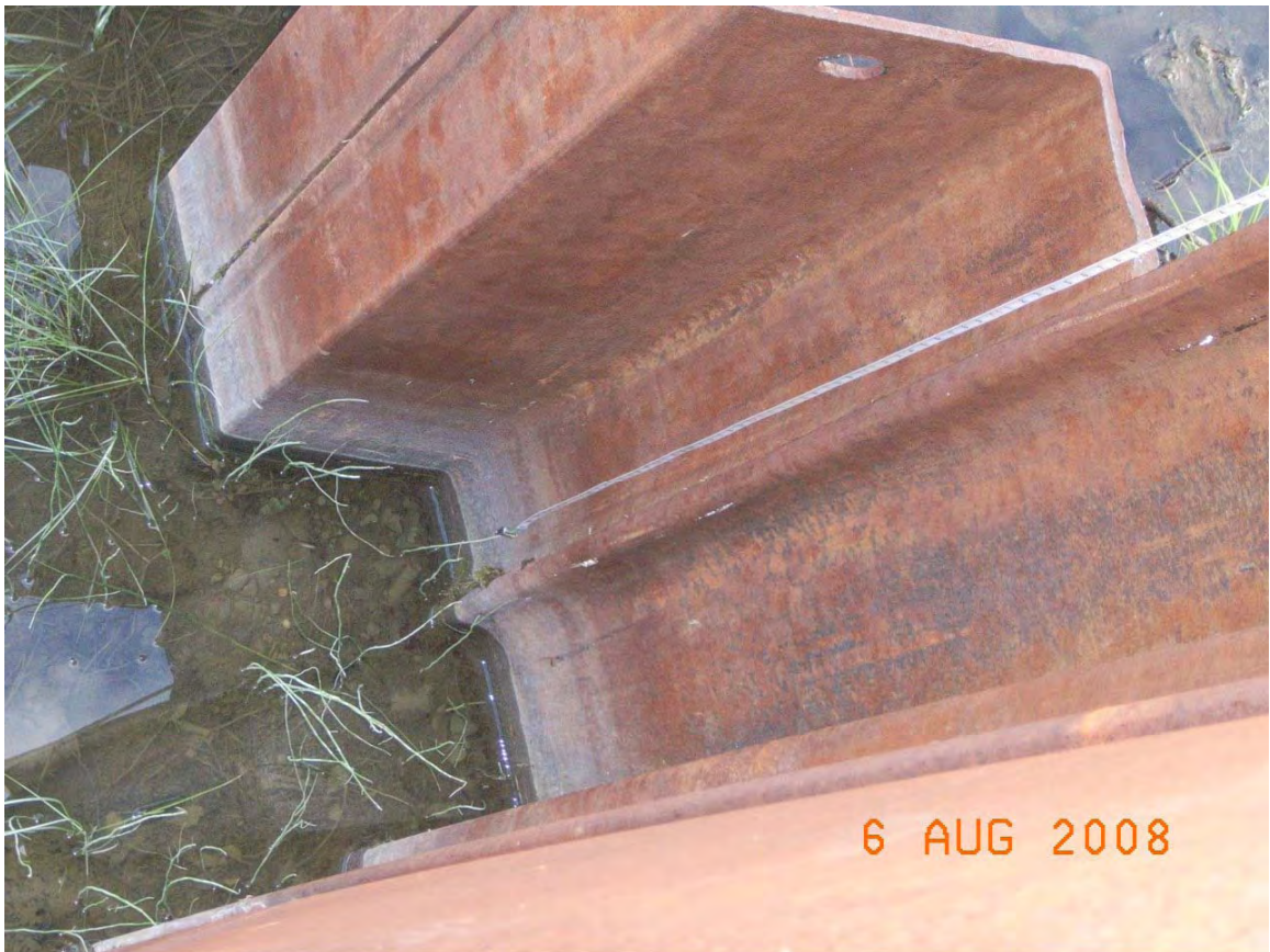
Figure 4: Silt line on sheet pile sill, Fair, Chena Flood Control Project, 2008.
