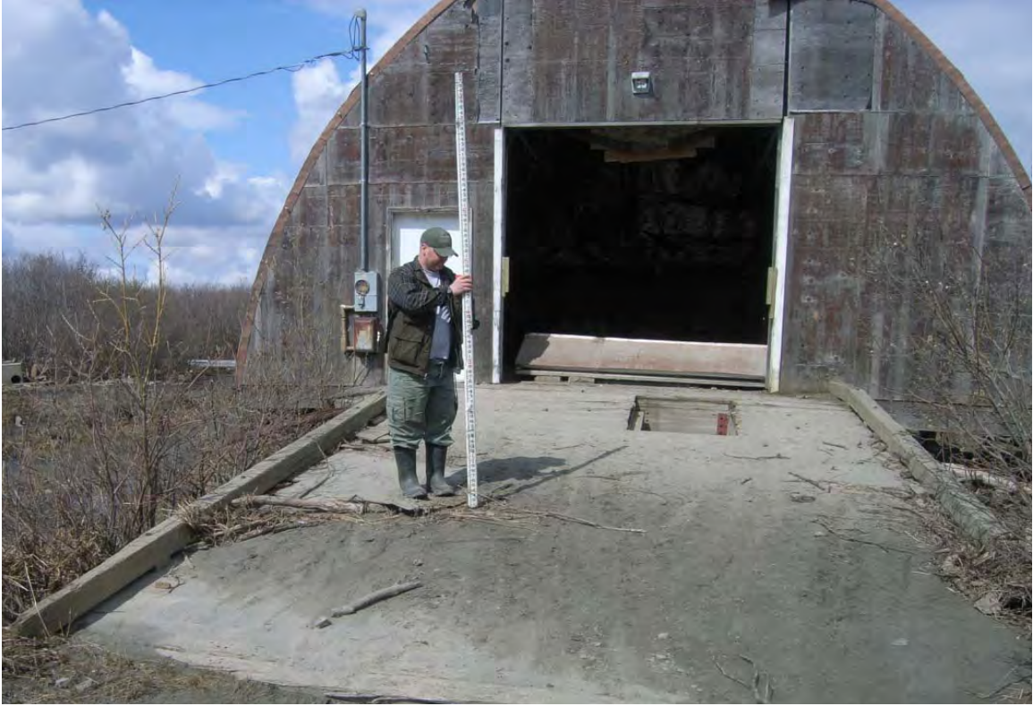
Figure 9: Debris line on access ramp, Fair. Emmonak, 2009.
