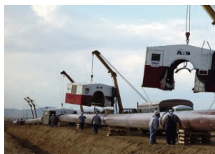
Kern River Pipeline
